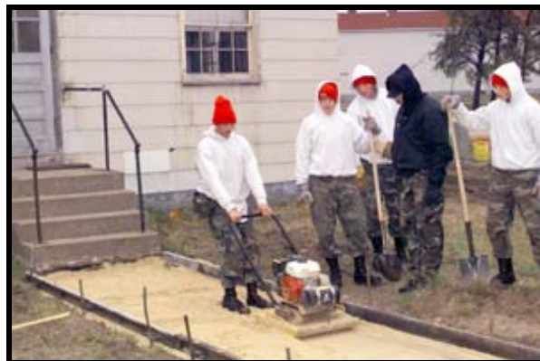
Cadets from the Challenge Academy at Fort McCoy, under the supervision of a Challenge Academy Cadre, work to put in a sidewalk in the front of the Challenge Academy headquarters (off Fort McCoy's website 9/04)
